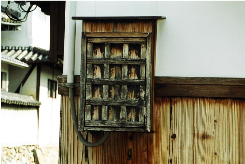
Utility meter box
