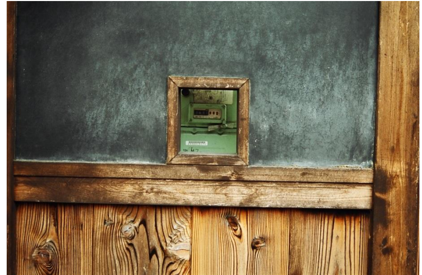
Utility meter box
