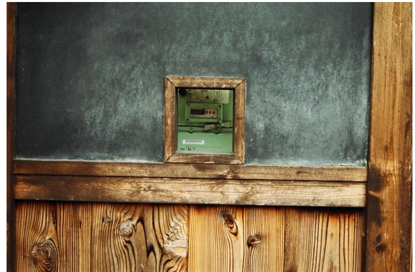
Utility meter box
