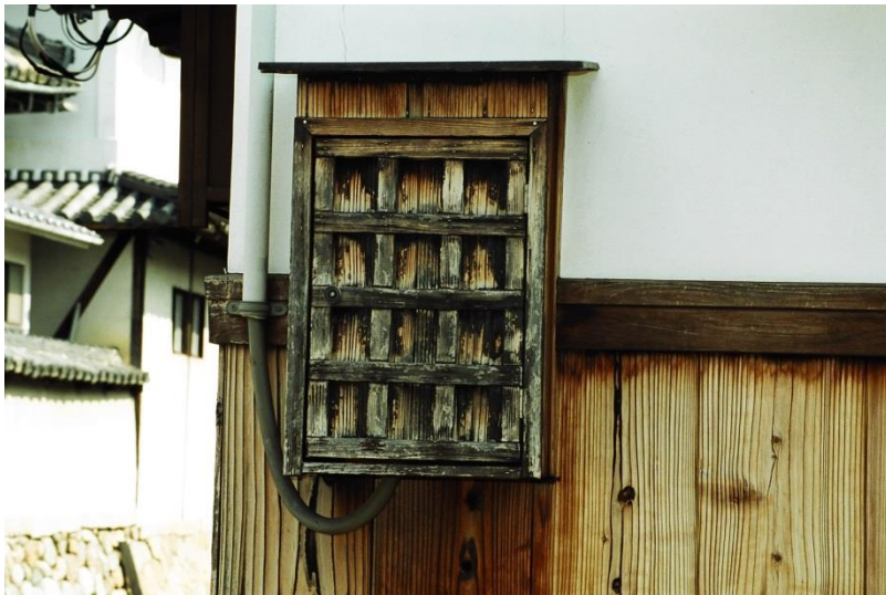
Utility meter box
